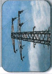
No High Tension Line
